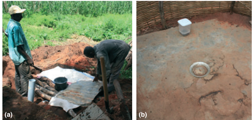
Figure 1 Construction of a latrine flytrap. (a) Here, a membrane is applied over a row of logs before concreting. In the centre is the bucket acting as a mould for the drop hole and to the left is the vent pipe on which the trap is positioned. (b) The completed latrine with drop hole cover and flytrap in place.
