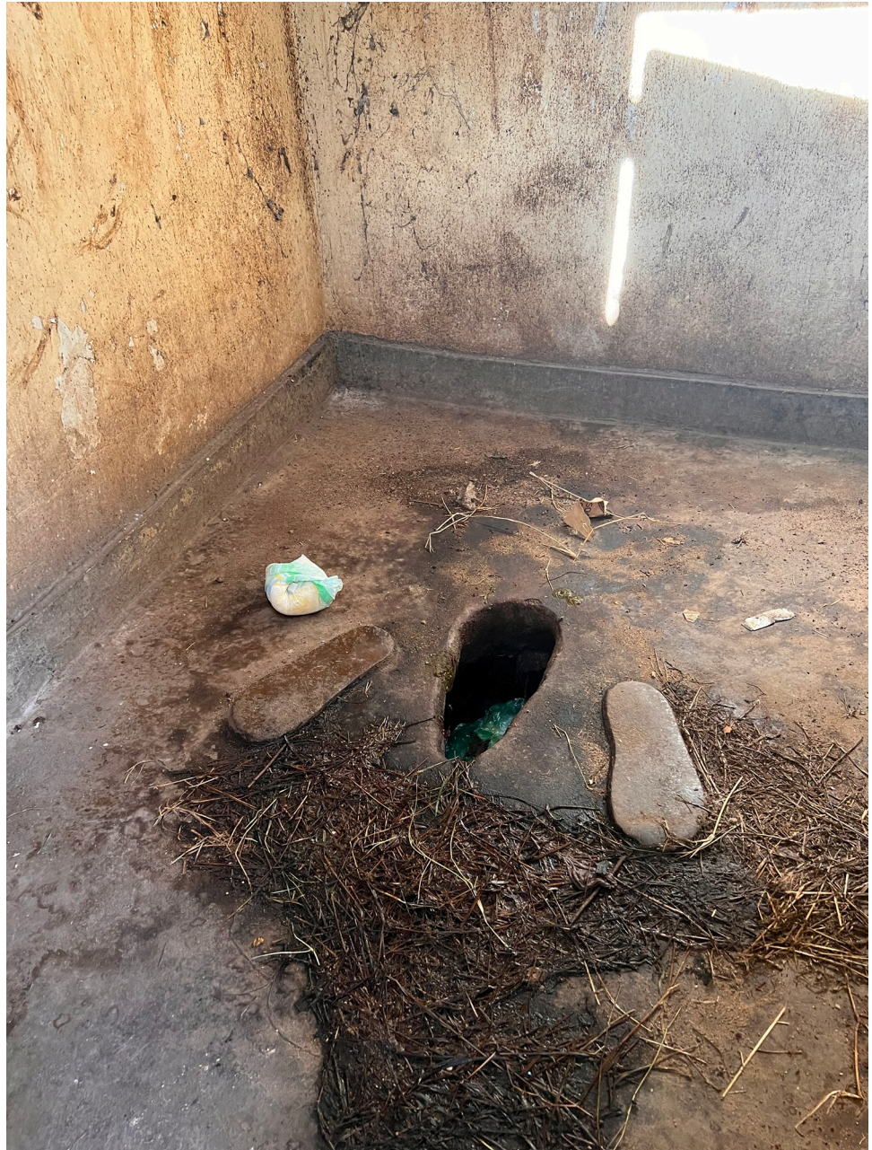
Fig 5. Guardian waiting shelter pit latrine, which is full, with indiscriminate disposal of diapers.
