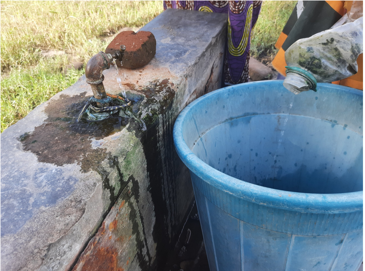
Fig 4. Broken water tap located within the Guardian waiting shelter.
