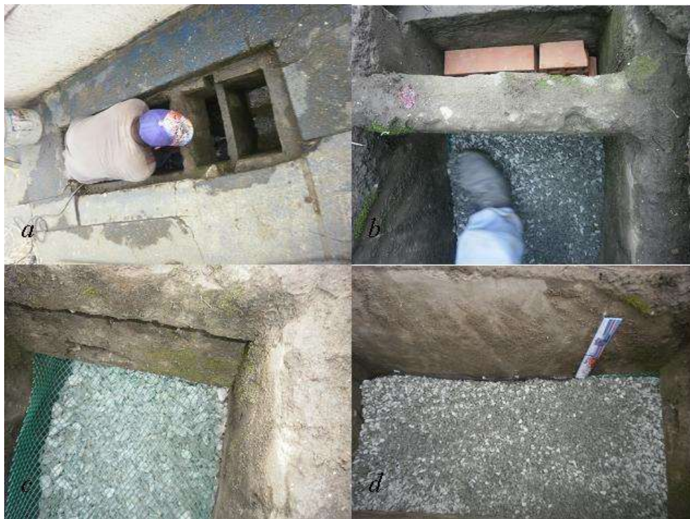
Figure 2. Storm drain modification process. (a) Screen perforation, (b) Installation of brick and gravel 9.5 mm diameter (3/4"), (c) Installation of the diamond mesh d. Modified storm drain
