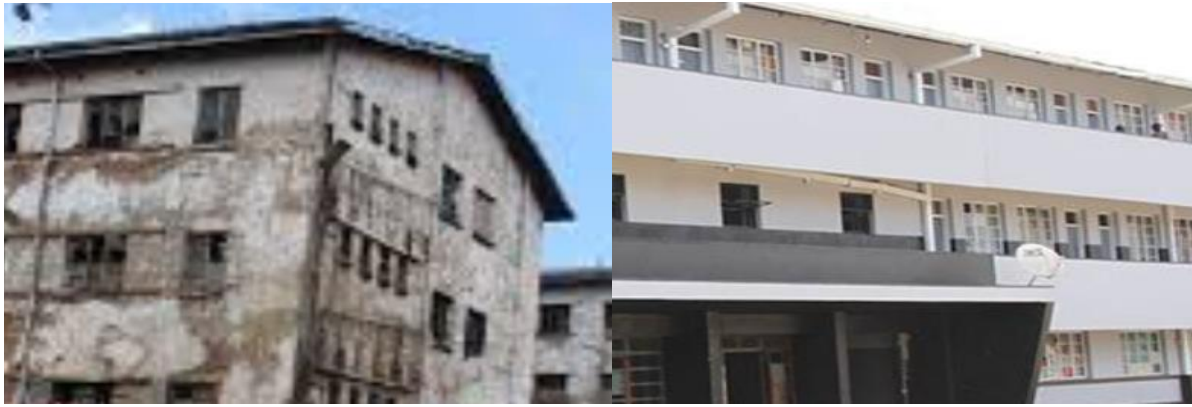
Figure 15: Matapi flats: Block not yet renovated (left) and block that has been renovated (right)
