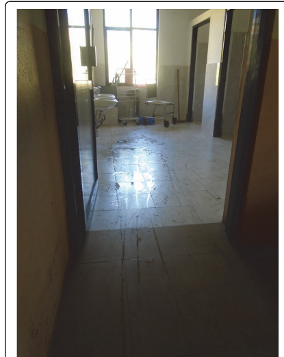
Fig. 4 "During period one should be careful using bathroom. Our legs might already feel weak so we might fall down and meet an accident. Here the toilets are made for everyone to use but if it was to built at home for crutches user, it is to be made in a way that it is not slippery. Marble should not be used as it is slippery." PhotoVoice image taken by BabitaThapa. Ranked 3 out of 5
