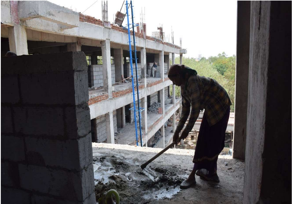
Photograph 1C: A female construction worker in Delhi working at a height without PPE and without railing
