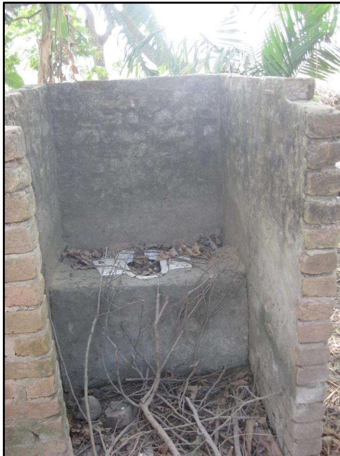
Figure 9. Badly built latrine in Bamanal village (Harijan sahi)
