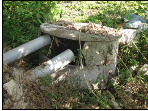
Figure 8. Broken latrine pit in Kajisahi village
