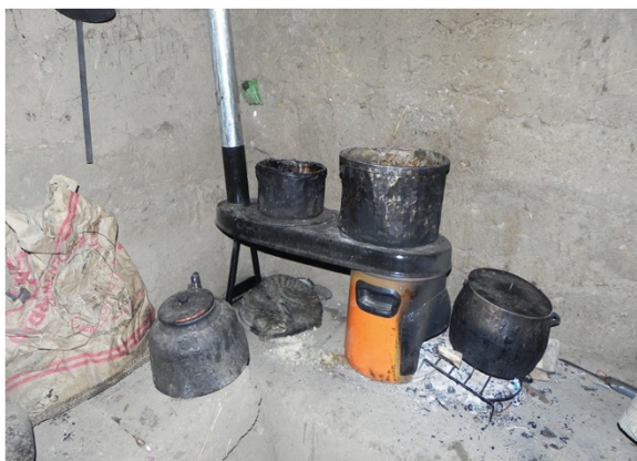
Figure 2 Envirofit G-3300/3355 installed in Peru.
